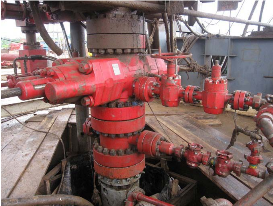
BOP stack up with 8500 psi under the blind ram
