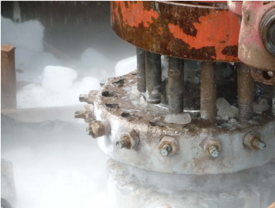
“Moment of Truth” BOP is lifted off the wellhead with only ice holding pressure
