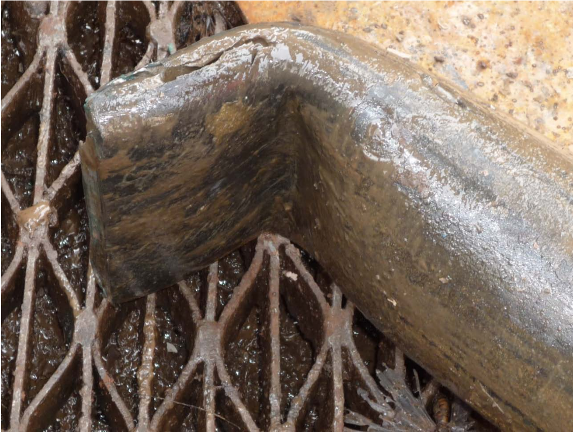
Top of sheared off landing joint (crimped during shearing – bent while fishing out)
