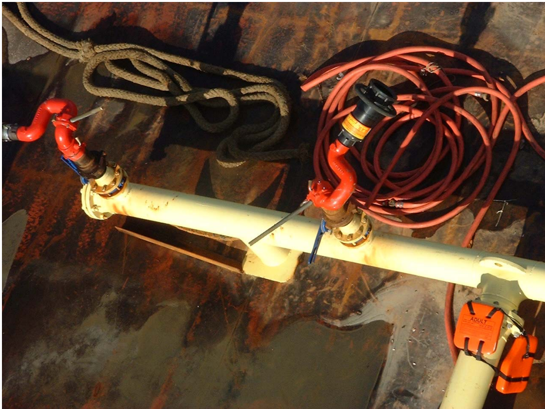
Figure 5.5 Marine Manifold On Offshore Location
