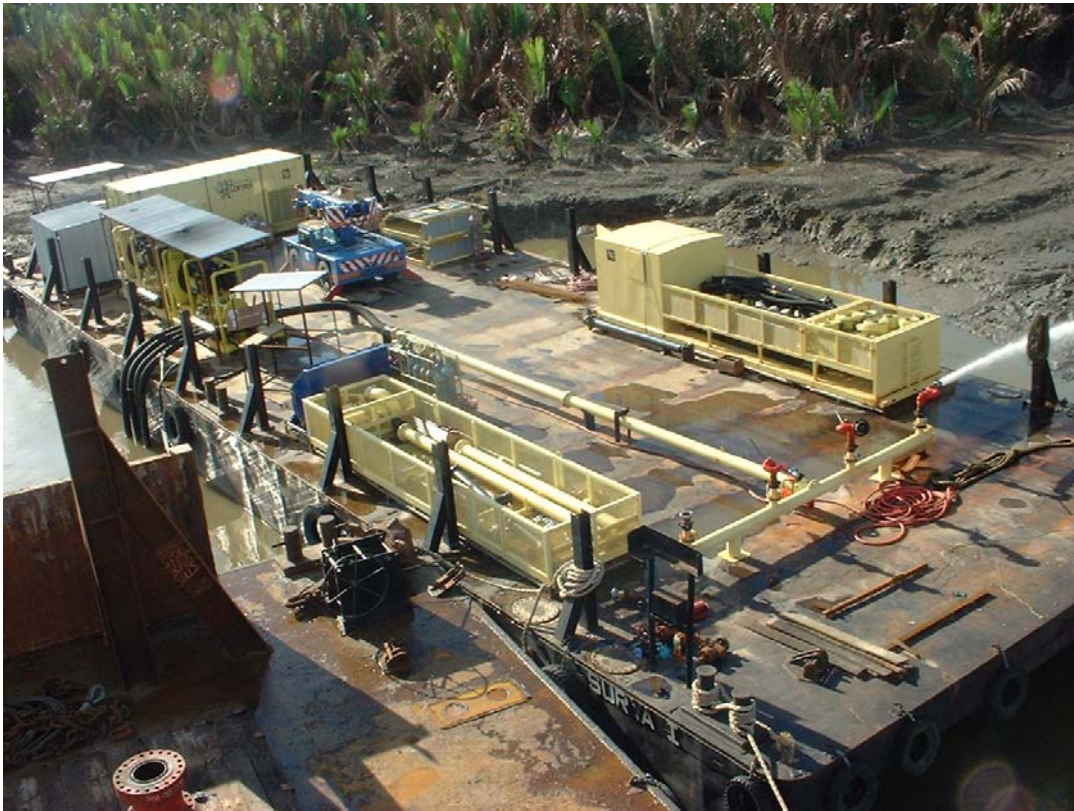
Figure 5.4 Crane Barge Firefighting Support
